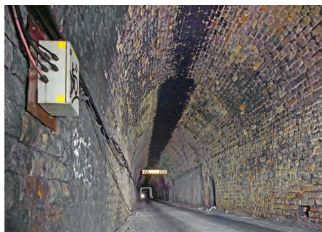
Nicholson railway tunnel showing the support vehicle's tyre tracks and one of the ceiling safety barriers at each adit.
